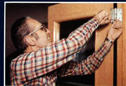
Gerry Schjelderup installs doors on outer lobby (doors had been missing for 30 years, were later found hidden in basement).
